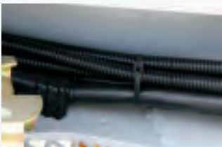
Air and electrical lines protected with automotive wire loom for optimal wire protection
